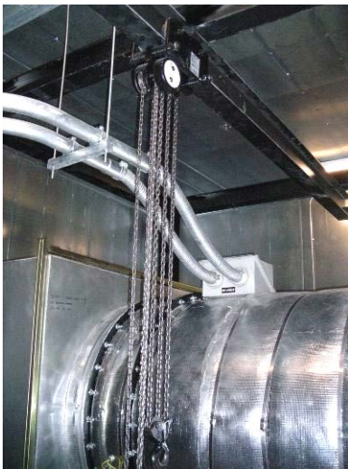
Large Motorized Fan and Overhead Hoist
