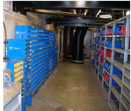
Spare Parts Storage
