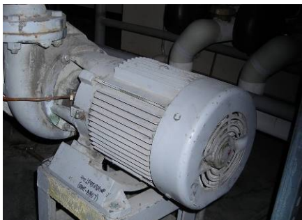
Example of Maintained Motor
