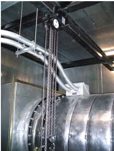
Large Motorized Fan and Overhead Hoist
