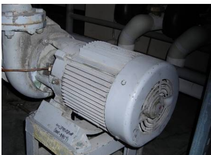
Example of Maintained Motor
