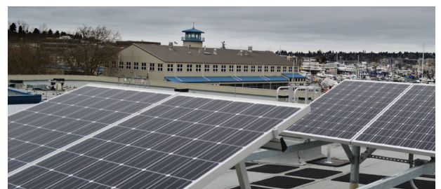
Fishermen's Terminal Solar Demonstration Project
