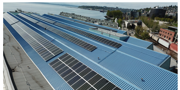
Pier 69 Solar Project
