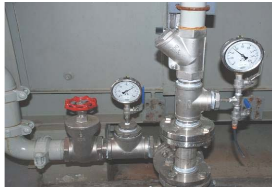
Valves and Gauges
