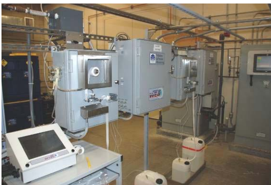
Water Testing Equipment
