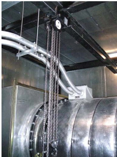
Large Motorized Fan and Overhead Hoist
