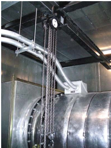
Large Motorized Fan and Overhead Hoist
