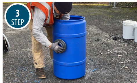
3 STEP Install 4-inch schedule 80 PVC bulkhead fitting in the hole drilled in step one.
