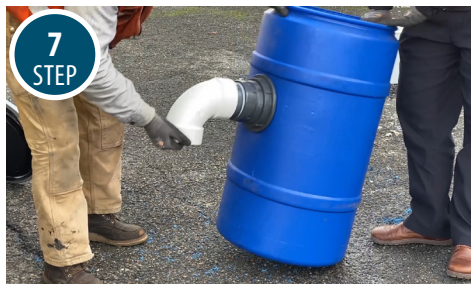
7 STEP Install 4-inch schedule 40 PVC 90-degree elbow downspout to the threaded nipple.
