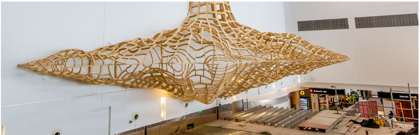
Installation of John Grade's Boundary as part of the North Satellite Modernization Project.
