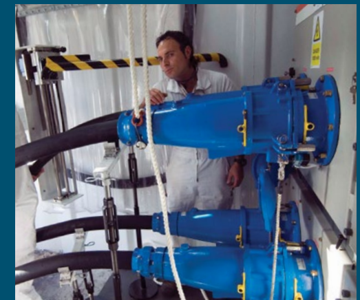
Shore power connections reduce emissions while at berth.
